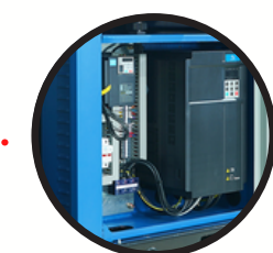
VSD Controller for Main & Fan Motor
